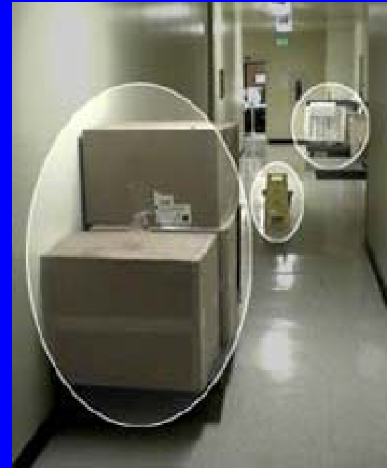
Obstructed exit route
