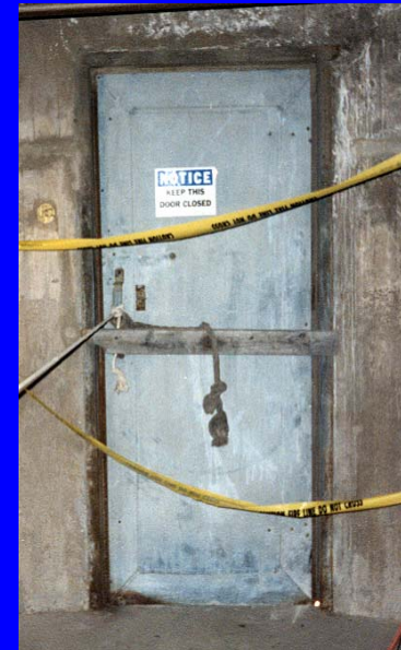
Locked and blocked exit
